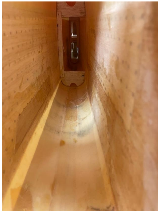
Photo 8: Looking aft inside the fuselage. More core repair and partial former repair. This was hard to reach!
