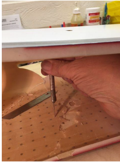
Photo 3: Removing damaged core and inner skin. Note the original epoxy filled core holes.
